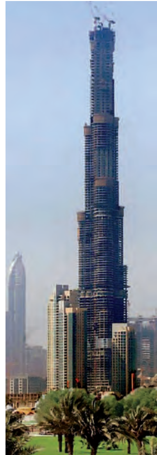
Burj Dubai, the tallest building in the world, under construction in October 2007.
